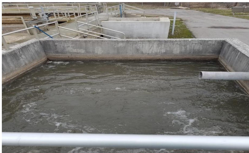
Figure 2-5 Aerated Grit Chamber
