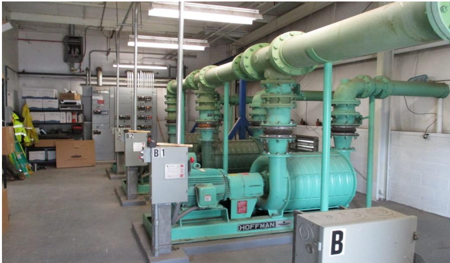
Figure 2-7 Centrifugal Blowers and Air Header
