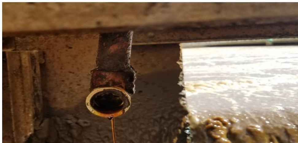
Figure 2-11 Ferric Chloride Feed at AT Discharge Point
