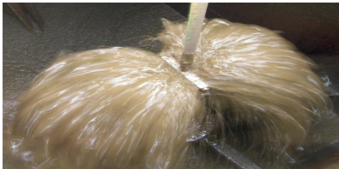
Figure 2-15 Telescoping Valve Flowing with RAS Biosolids
