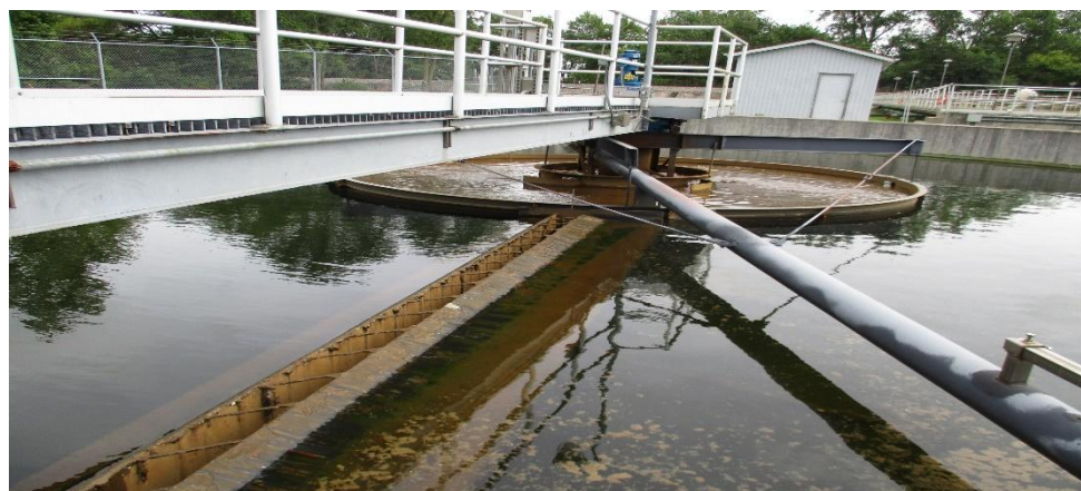
Figure 2-13 Secondary Clarifier in Service
