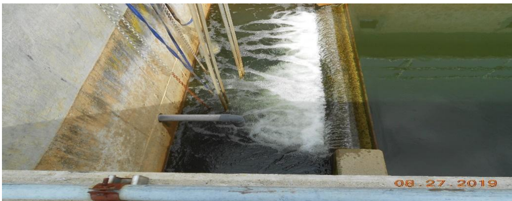
Figure 2-19 Dechlorination at Discharge of Chlorine Contact Tank
