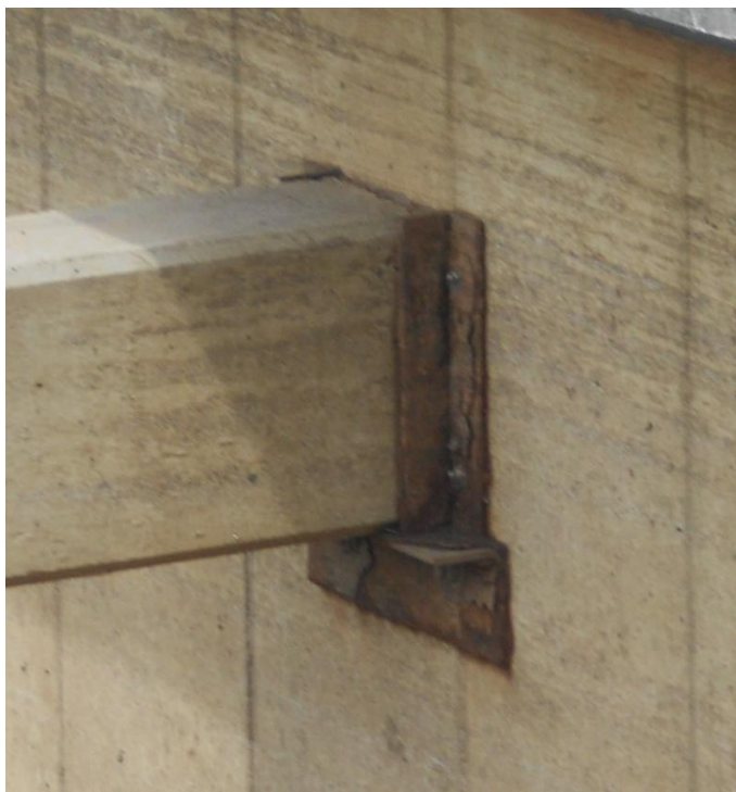
Figure 2-9 Rusted Steel Beams Supports
