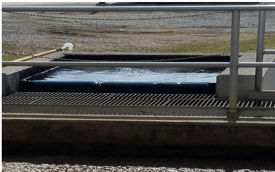
Figure 2-10 Industrial Forcemain Discharge Point
