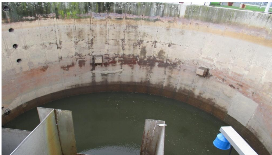
Figure 2-22 Old Anaerobic Digester Converted to EQ Basin
