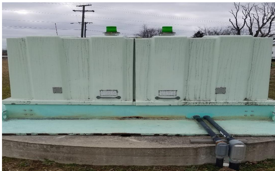
Figure 2-4 Wet Weather Pump Station
