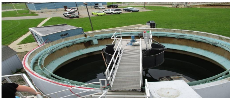
Figure 2-23 Clarifier Converted for Wet Weather Primary Clarification
