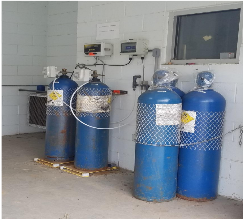
Figure 2-17 150 # Chlorine Gas Cylinders
