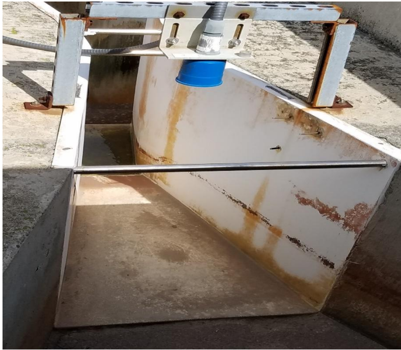
Figure 2-24 Parshall flume and Transducer for Wet Weather Flow
