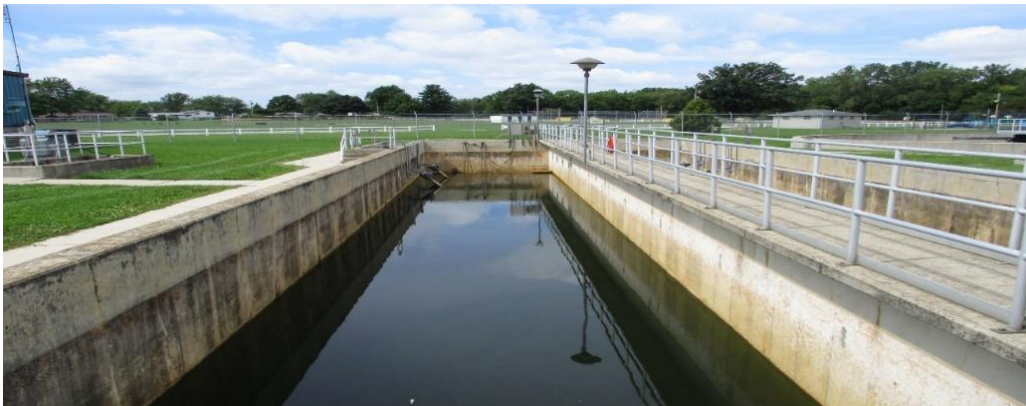
Figure 2-18 Chlorine Contact Tank, with Mechanical Aerators at Discharge
