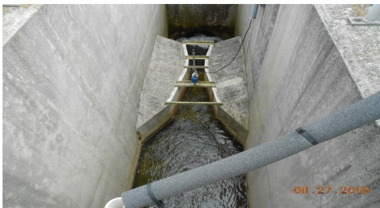
Figure 2-20 Parshall flume and Level Transducer for Effluent Discharge to Outfall 002
