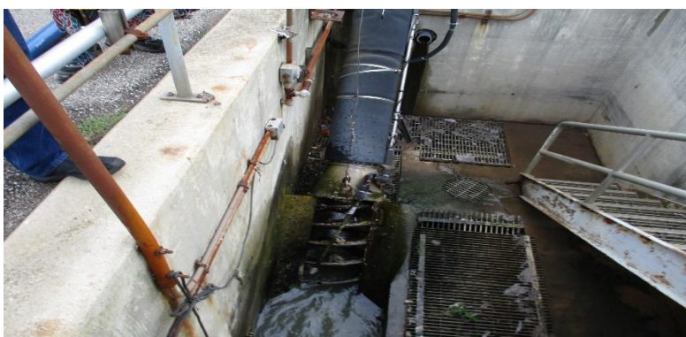
Figure 2-2 Rotary and Bar Screens
